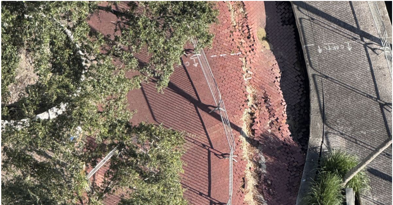
The barricaded section of Riverwalk North seen from above, with the brick walkway sunken and pulled away from the seawall. Photo: Nathan Stevenson, 2026.
